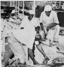
A GROUNDING system is installed by workers, above left. Others smooth poured cement before the ditch is filled, braze cables going through into the government substation grounding system, and build pull boxes through which Lago's power cables will be connected to government switching gear.
